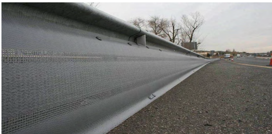
View of the installation in the city of Madrid on the road A1 Madrid in November 2007.
